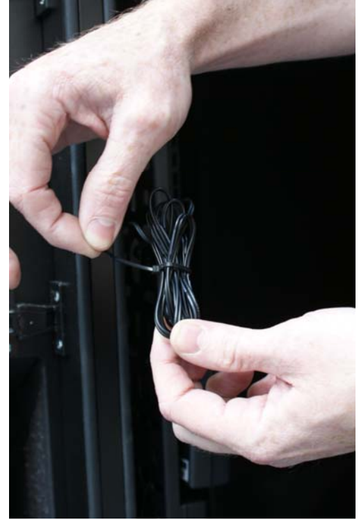
3. Tidy the excess jack-cable into a bundle, hold together with the small cable-tie and tuck behind.
