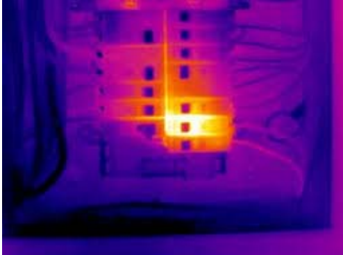
Figure 1: Infrared Scan showing Normal Temperatures of Circuit Breakers in a Load Center
